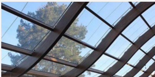
Figure 5: Building-Integrated Photovoltaics: Acting as both cladding & Solar generator
